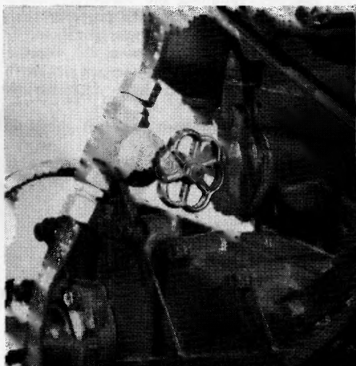
Fig. 8 The water by-pass gate valve
